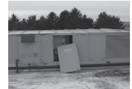
40-year-old heating/cooling systems
